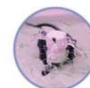
循环水泵 Circulating Water Pump
