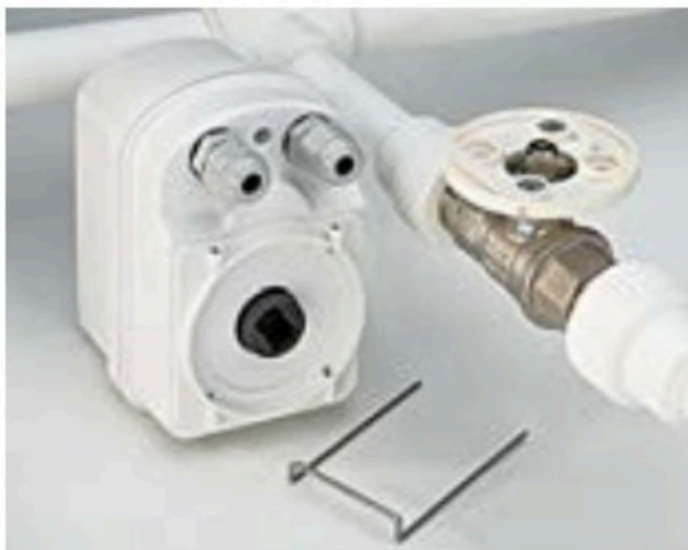
Photo 1. Ball valve and electric actuator
