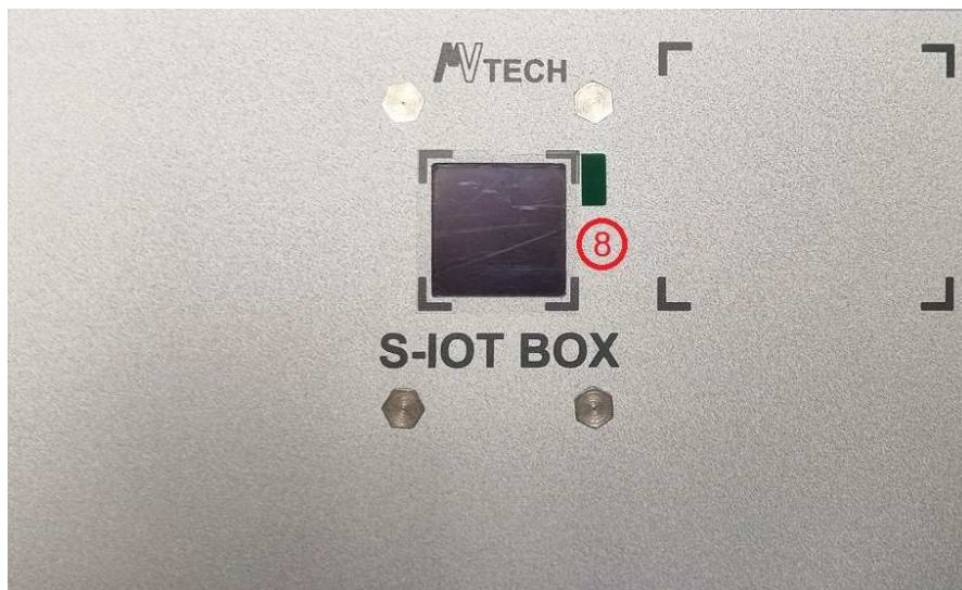
(IOT_4_VIBRATION TOP Exterior)
