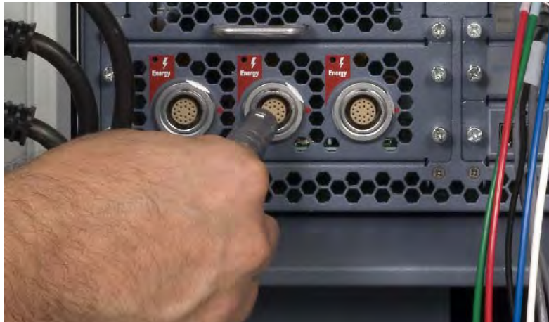
Figure 4.14 Auxiliary device connections (back of Core)
