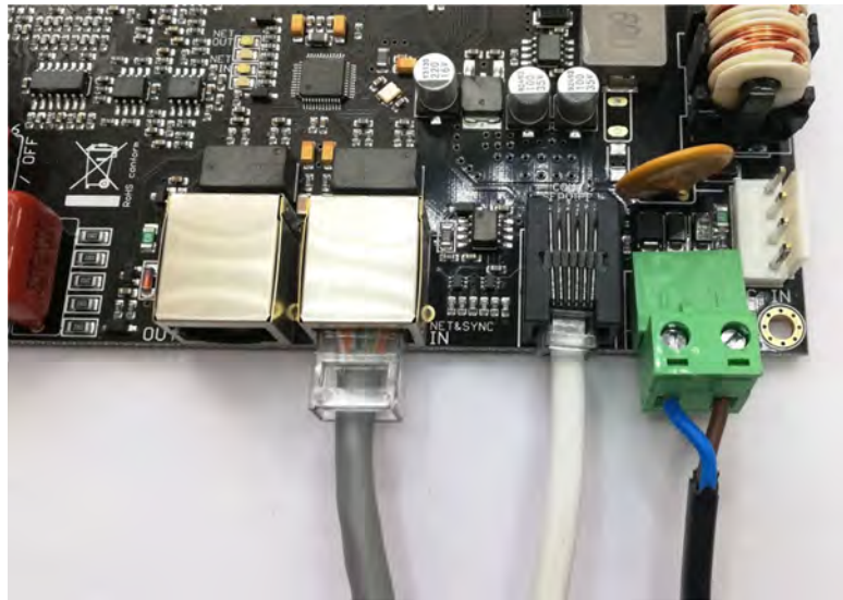
Picture 2 - Connected el. board
