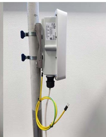
Installation the Wirnet™ iStation on the support
