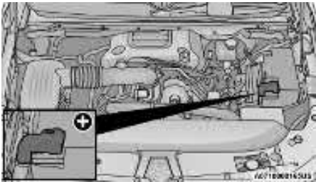
Positive (+) Battery Post Location
