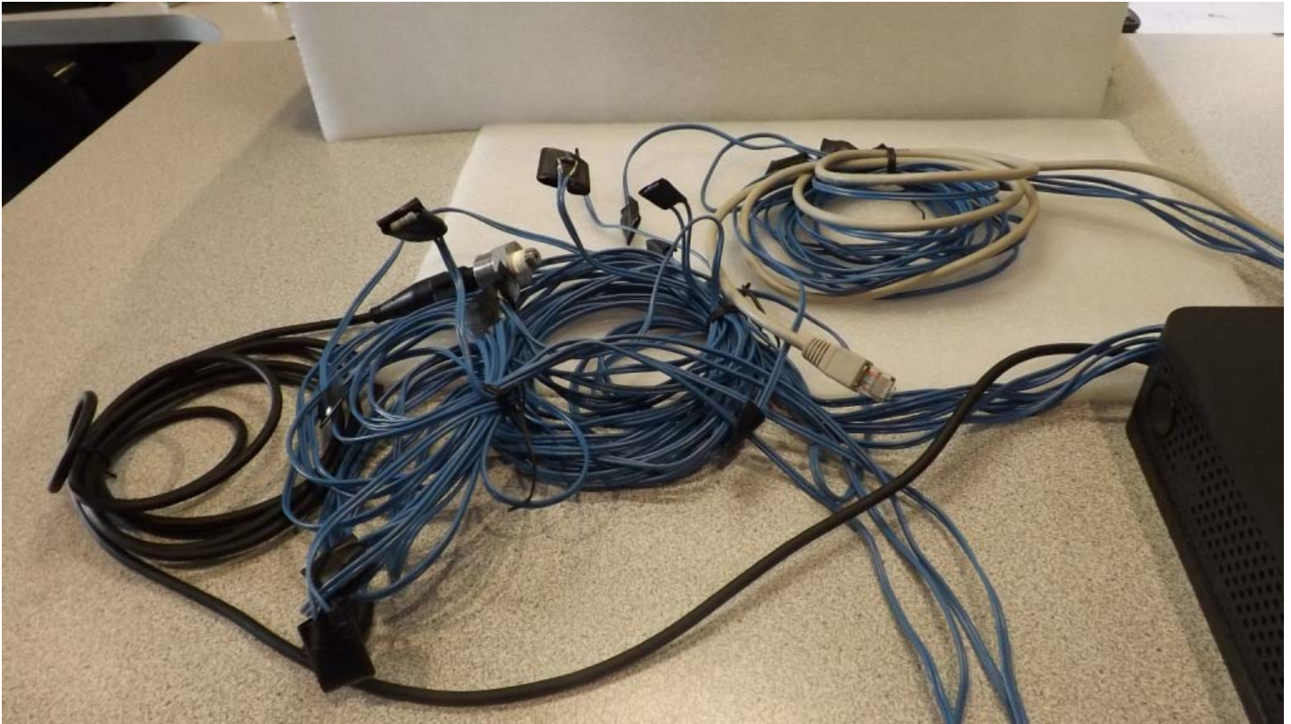
Figure E23.9 – Setup – Cable Terminations
