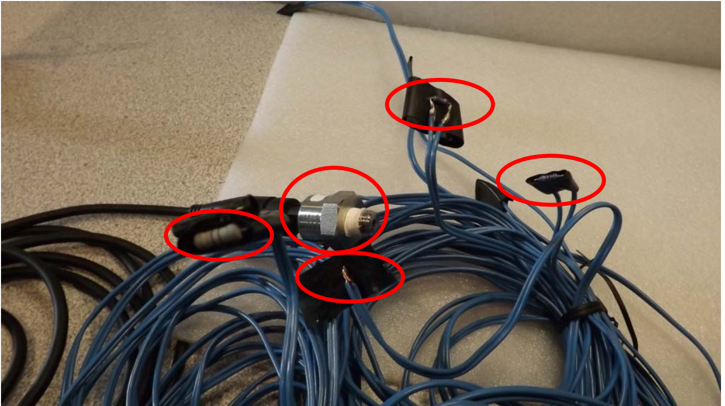
Figure E23.10 – Setup – Cable Terminations
