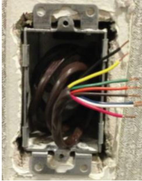
Fig. 2 -- Coil Excess Wiring
