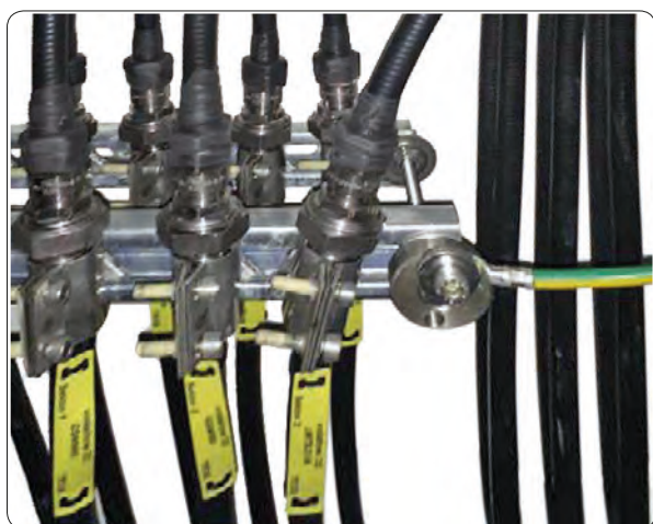
Fig. 2: Example of a handover point for the BTS signals at a c-rail
