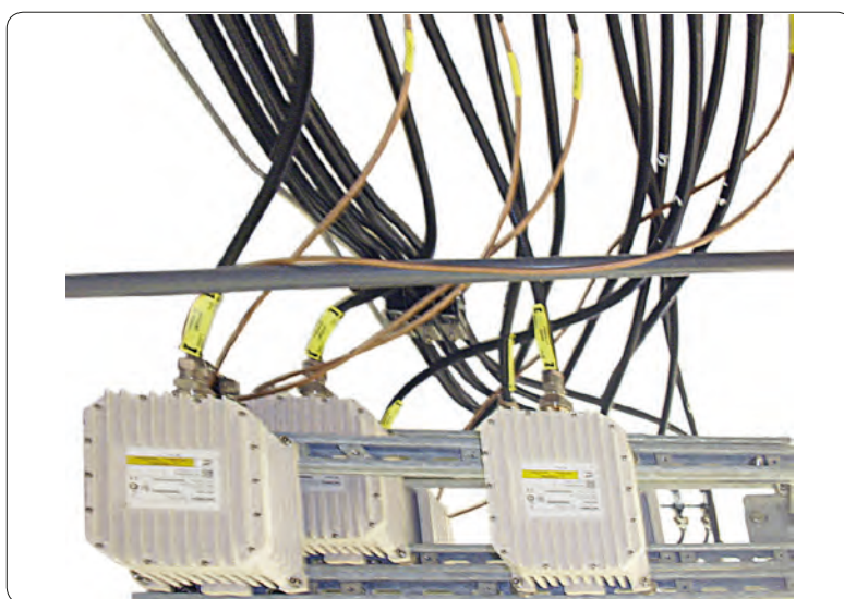
Fig. 3: Example of a handover point for the BTS signals with individual loads with short patch cables at a c-rail
