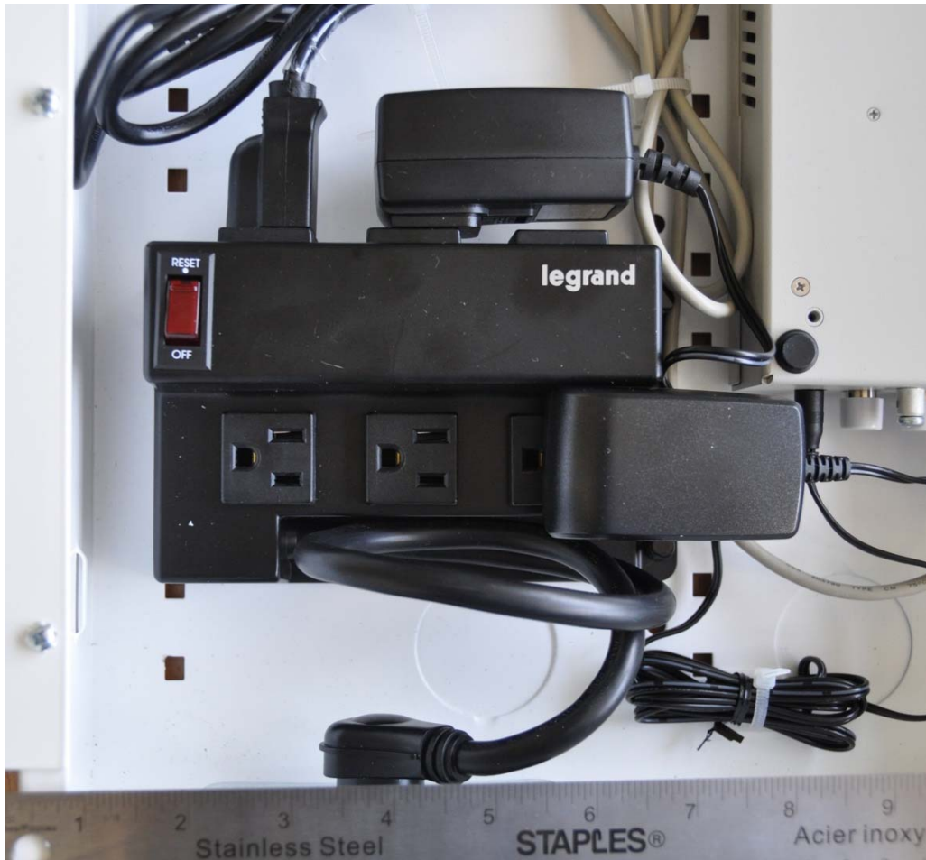
Figure 4 - Power Bar (Within Service Box)
