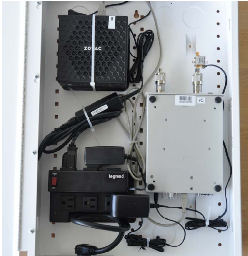
Figure 1 - Service Box Interior
