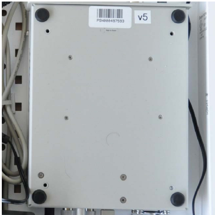
Figure 5 – P148 Transceiver (Within Service Box)
