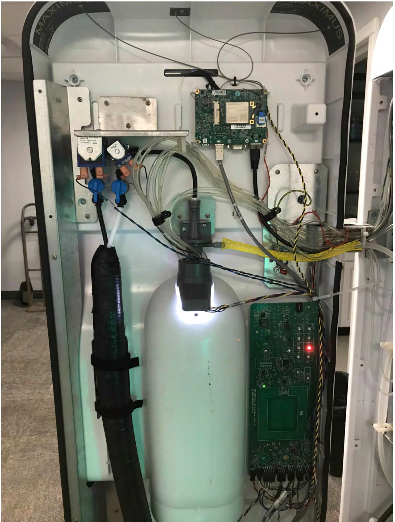
V2 Machine Inside Door View Closeup
