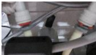
Pump 1 Cable at Pump Ferrite PN 046178181
