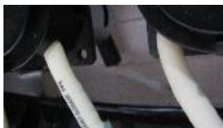
Pump 3 Cable at Pump Ferrite PN 046178181
