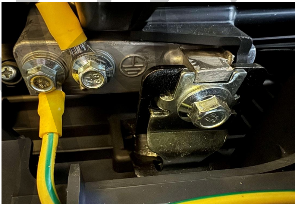
Photo 16 - Ground terminal bus
