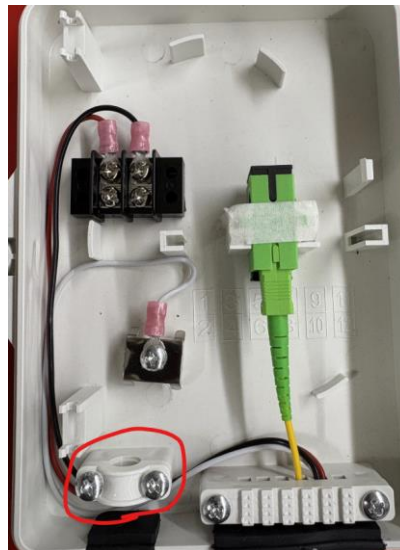
Figure 6: Location of the Hybrid Cable bracket in the fiber optical patch panel
