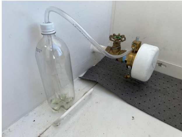
Figure 21: DGA-LT1 Ready to Bleed Air from Unit
