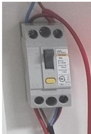
a power circuit breaker
