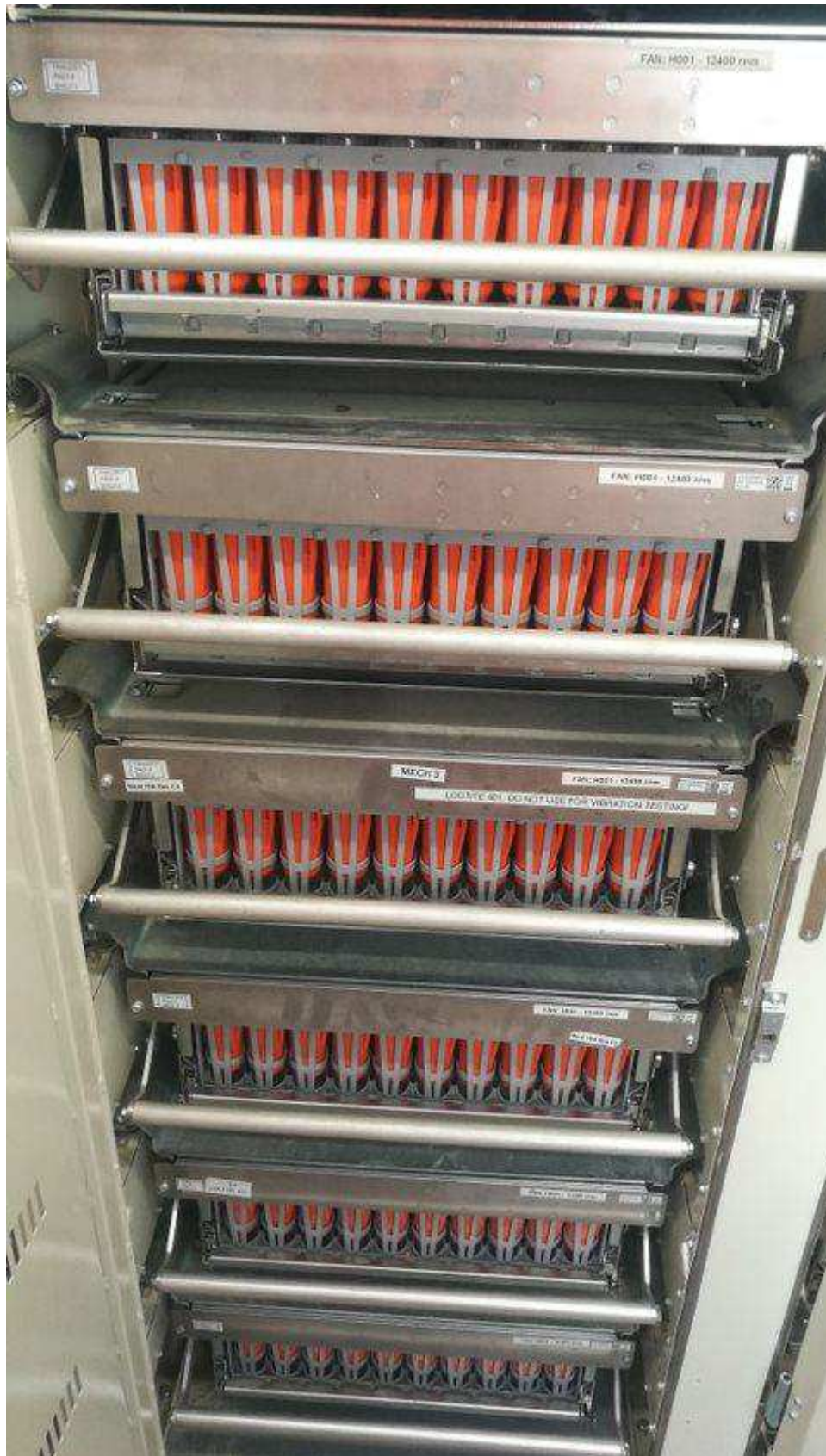
Nest Rack interior with charging shelves
