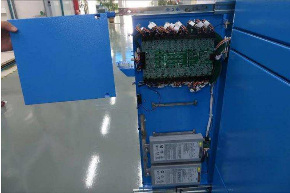
Internal view with 2pcs batteries
