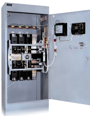
ASCO (Schneider Electric) Series 7000 ATS(600A, 480V) Bypass-Isolation Switch
