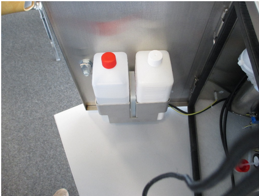
Picture 7 Installed CCM10404715
