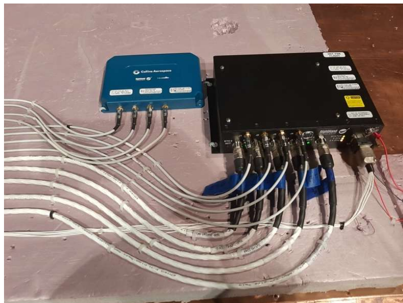
CabinLink Antenna Cabling
