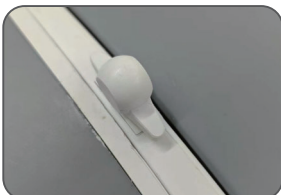
Water tank cover unlocked
