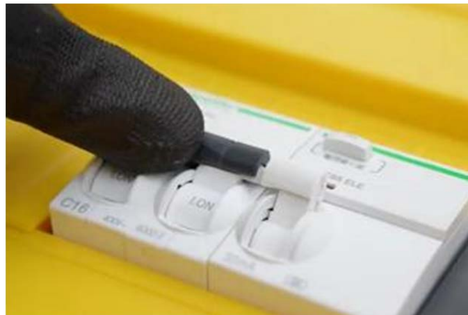
Fig 7.3 Air Breaker Check
