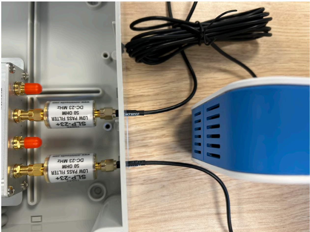
RFID reader in cabinet with no lid, close up picture of low pas filter mounted between HF RFID Shielded Antenna EA2602-BL-P & HF RFID Reader RD 2104.
