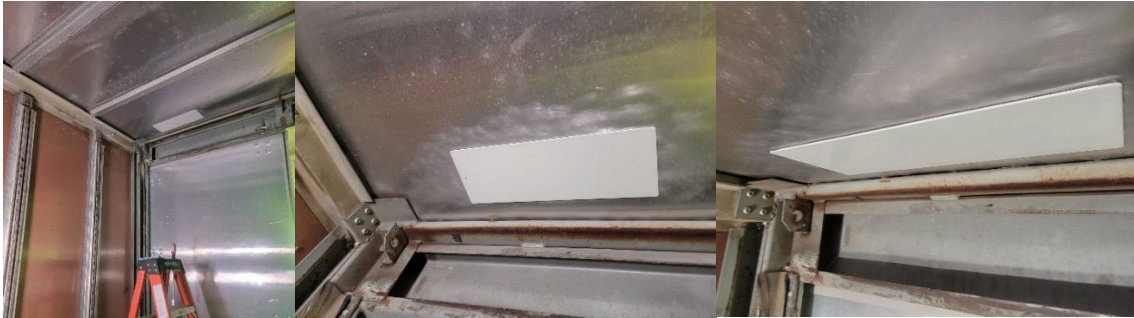
IU Mounting Plate Installed in a Trailer
