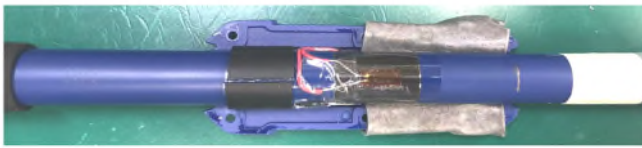
Photo from bottom (half removed adhesive tape)
