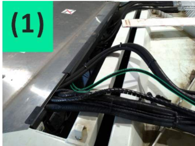
Cable tray from hopper to roof
