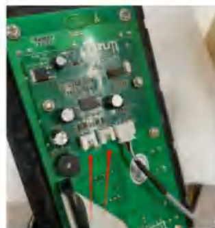
Check the wires behind the control panel
