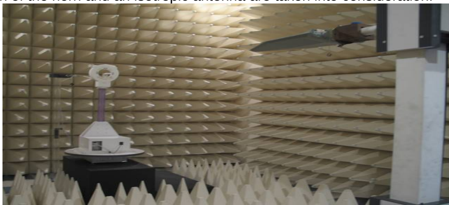
Figure2. Photograph of 3m Fully-Anechoic Chamber
