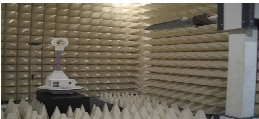
Figure2. Photograph of 3m Fully-Anechoic Chamber
