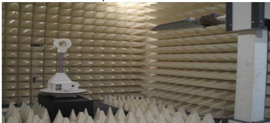
Figure2. Photograph of 3m Fully-Anechoic Chamber
