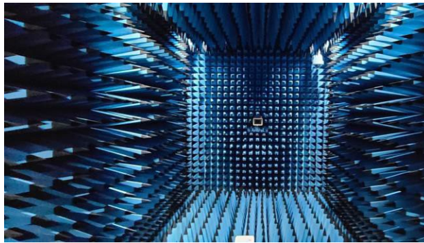
Figure 2: Geometry of Anechoic Chamber for Radiation patterns.
