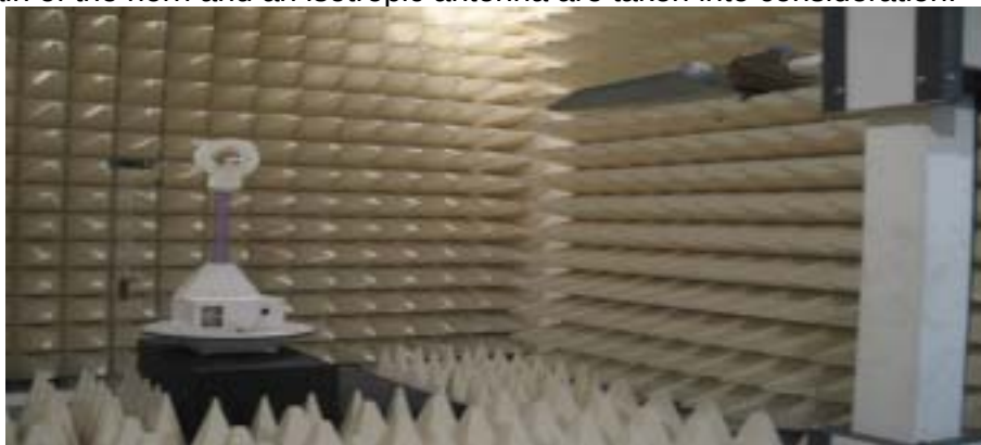
Figure2. Photograph of 3m Fully-Anechoic Chamber
