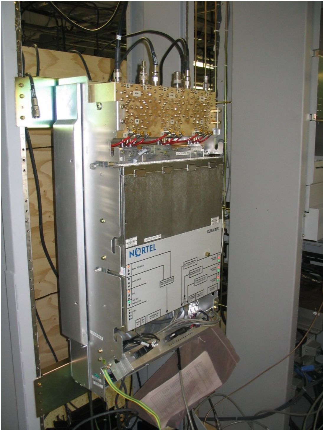
Nortel Networks vBTS 3030 Left Front Side View With Cover OFF
