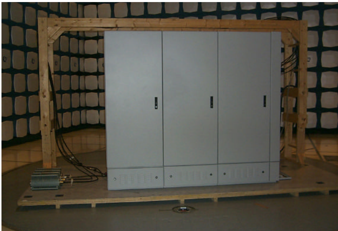
Figure 1: Front View of TDMA 800MHz Enclosure System
