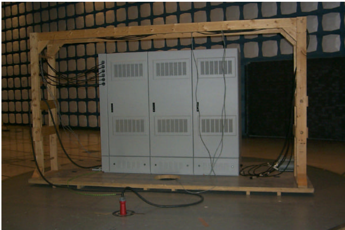
Figure 3: Rear View of TDMA 800MHz Enclosure System
