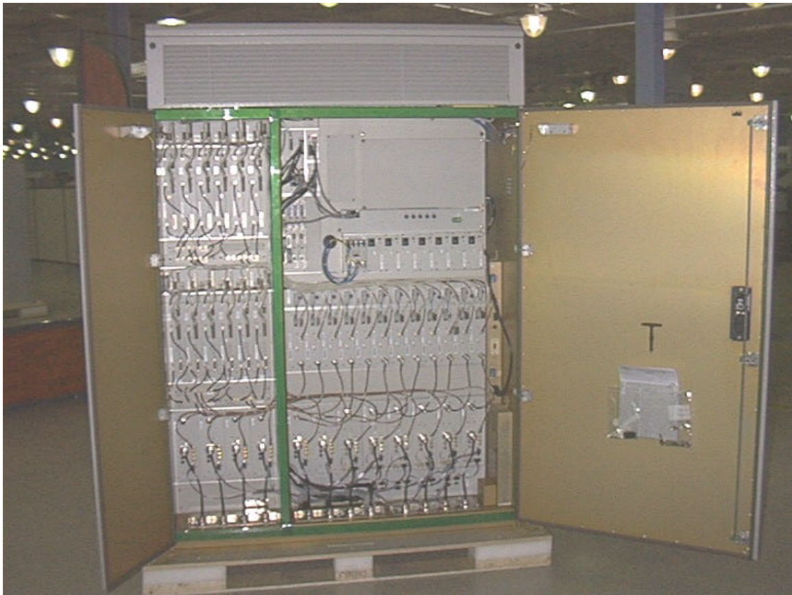
Figure 2 – S12000 Outdoor Front View with Doors Open
