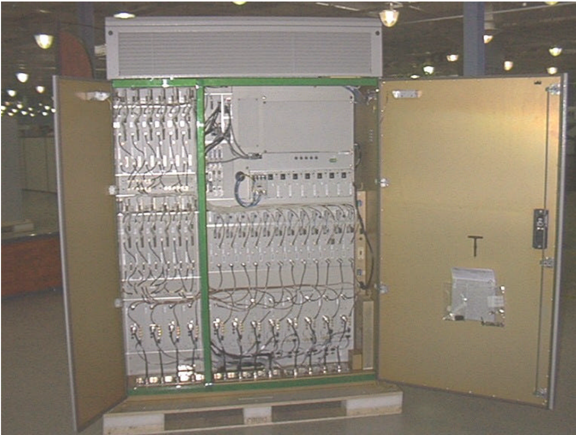
Figure 6 – S12000 Outdoor Front View with Doors Open
