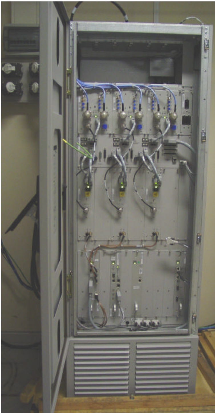
Figure 2: UMTS 1900 Front view with door open
