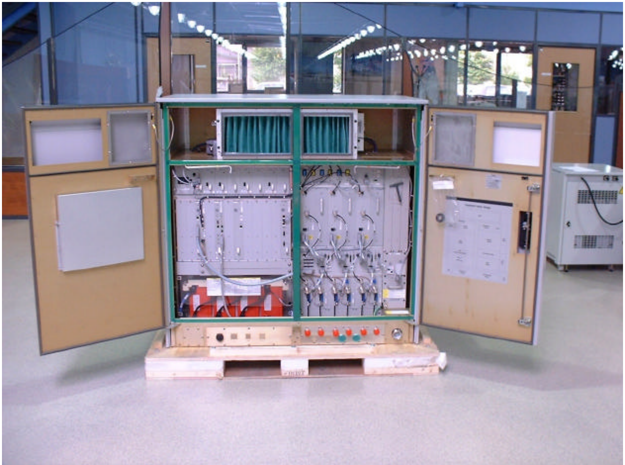
Front View, doors opened
