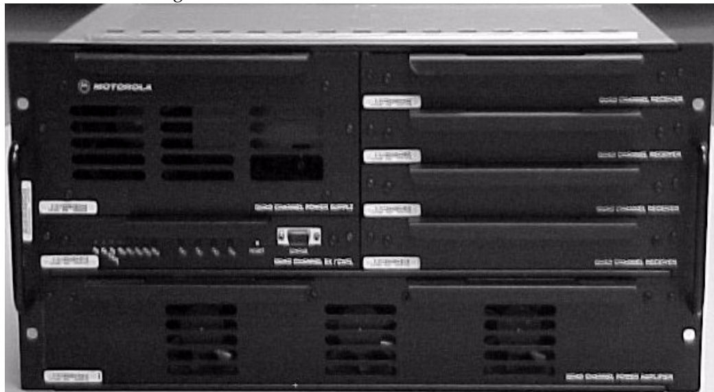
Figure:1-2 QUAD Channel Base Radio (Typical)
