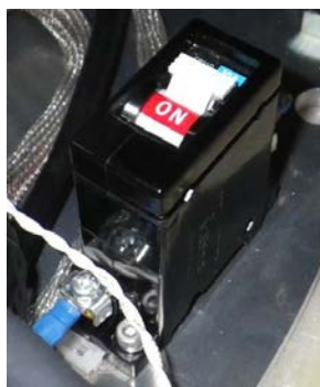
Antenna rotary motor switch "ON"
