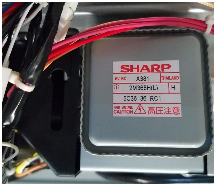
Figure 1. Close-up of Magnetron Label in situ
