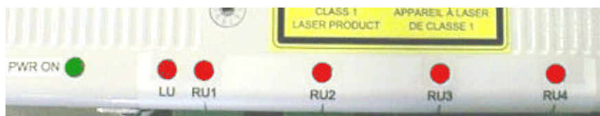
Figure 5 TFLF Local Unit Status LED's
