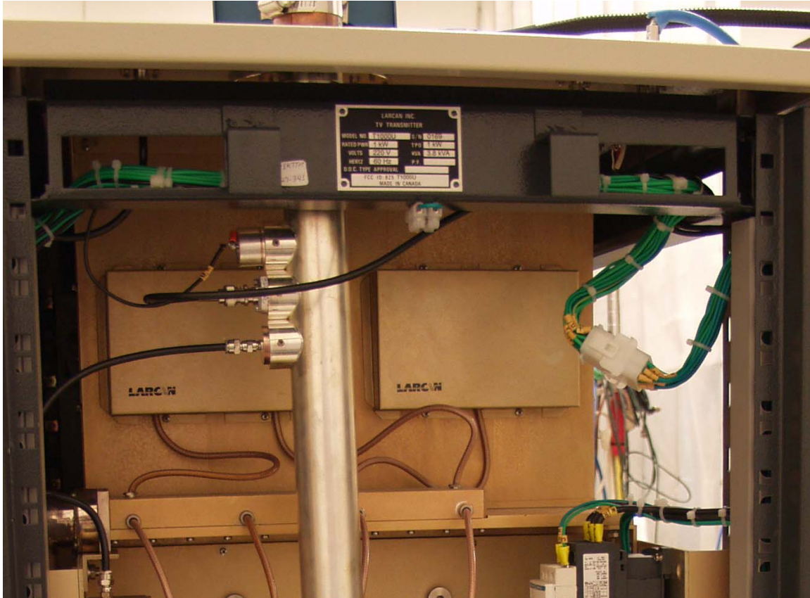
Label location at top rear of cabinet
