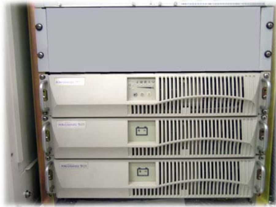
UPS System Front view
