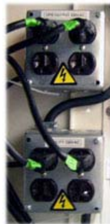
UPS & Utility outlets (rear side of cabinet)
