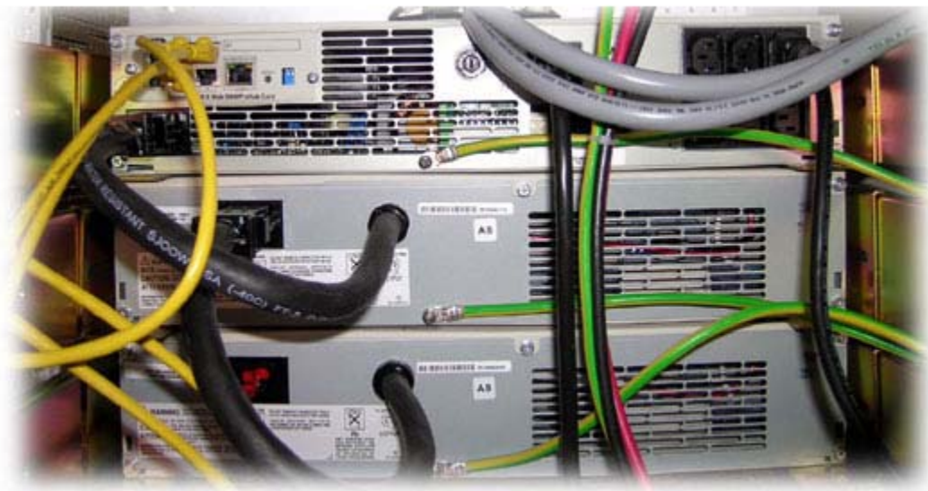
UPS System Rear view
