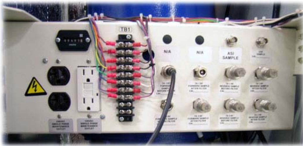
AC Distribution System Panel with AC Hour Meter and IF and RF Sample points
