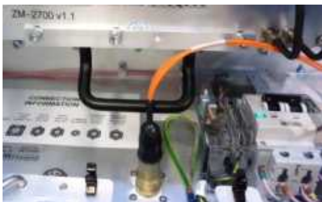
Fibre cable and connector restricting access
