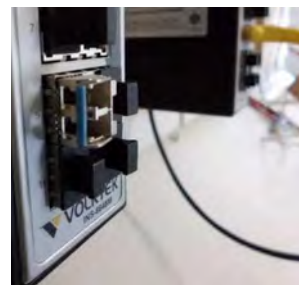
SFP module Installed
