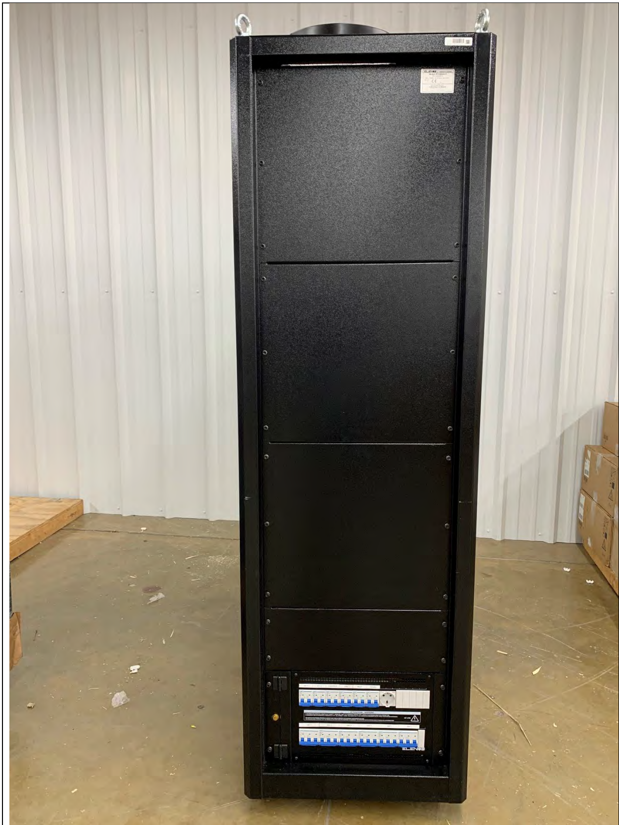
ET30000 In Rack Rear
